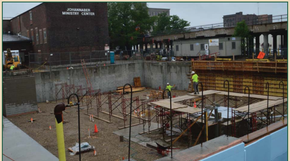
Progress even in the rain. June 11, 2014. Next they will pour the last foundation wall on the west and pour the basement floor. Set 2 beams, install the stairs and we will be ready for the pre-cast first floor. Progress!
